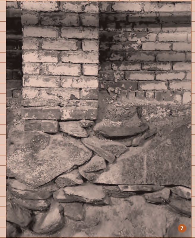
Students observed sectional material assemblies and abandoned "waste" brick in the underground portion of the former American Printing Company.
